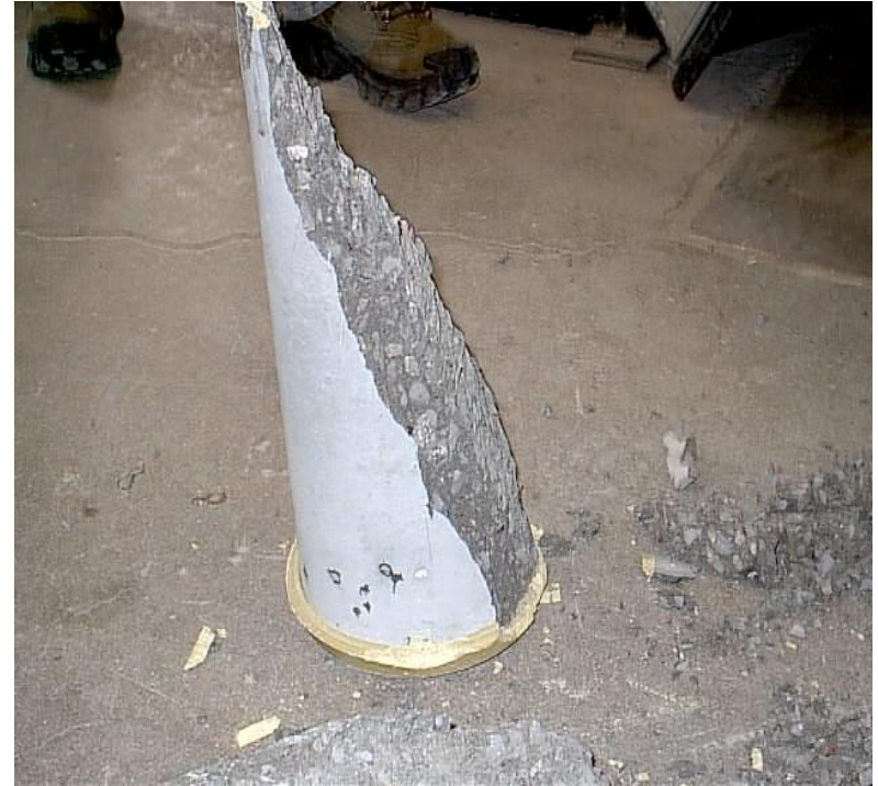
Failure in shear
