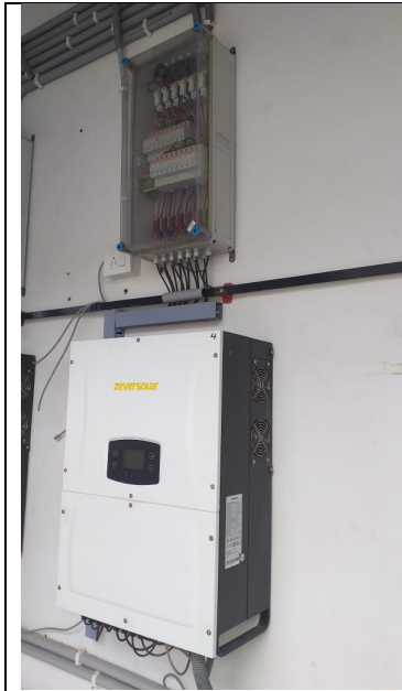
Solar PV Inverters
