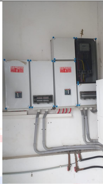
Solar PV Inverters/
