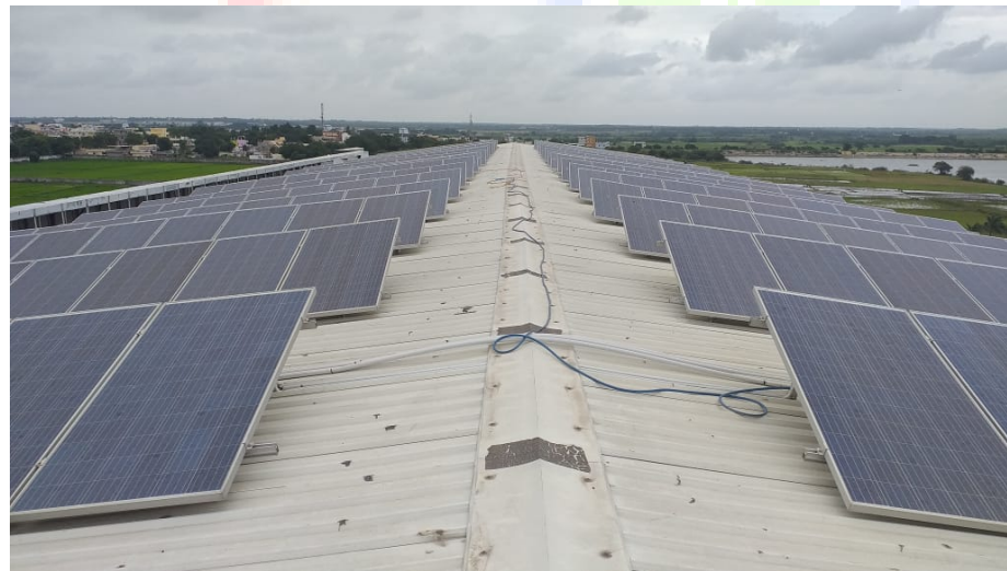
Solar PV Panels on roof top
