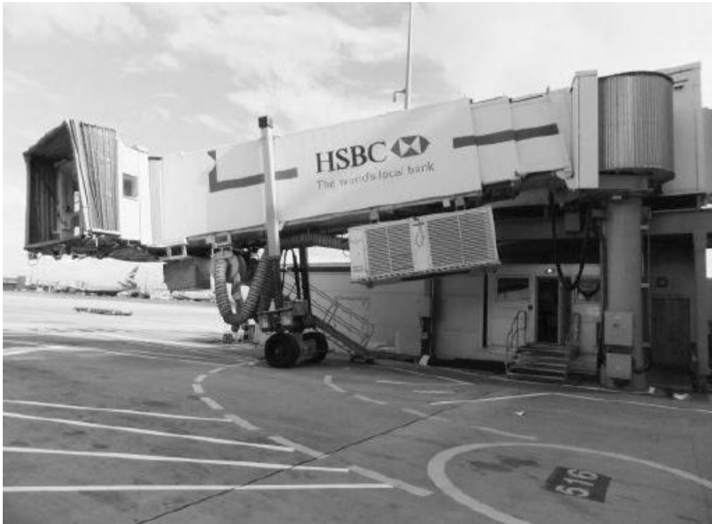
Fig 2.12 Fixed ground cooling unit attached to an air bridge
