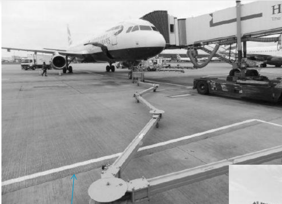
Apron cable electrical supply
