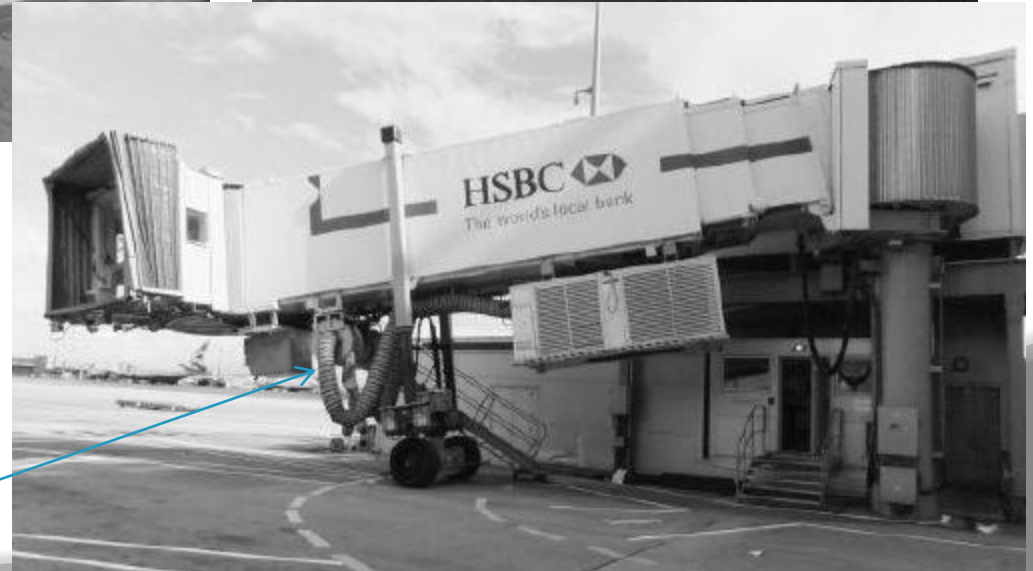
Fixed ground cooling unit attached to an air bridge
