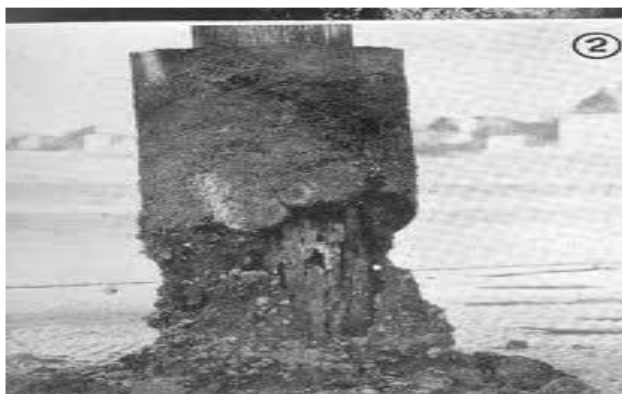
Fig. 1 Deterioration of concrete cover
