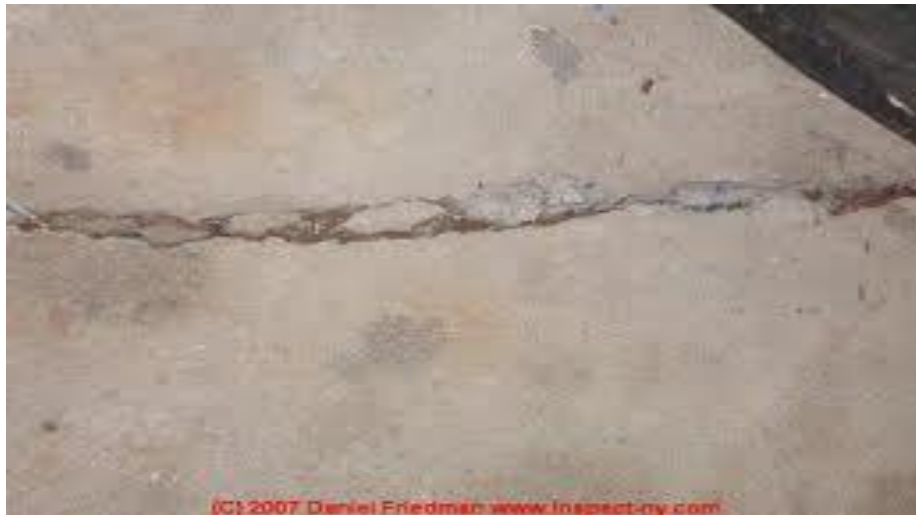
Fig.1 Cracks due to Early Frost Damage
