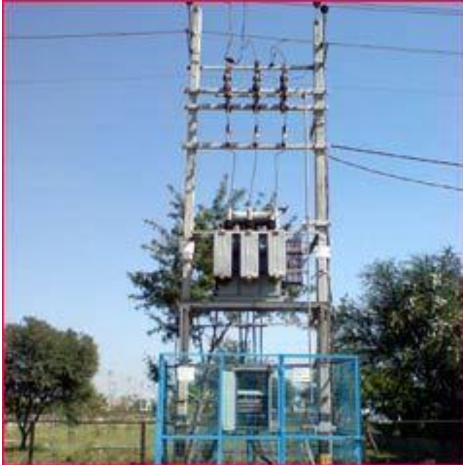
Fig. Outdoor Transformer
