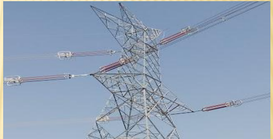
Fig.2: 765 kV transmission line in India with 4 sub-conductors per phase (Quadruplex bundle).
