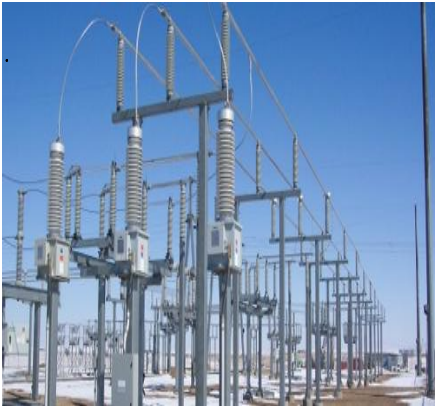
The electrical substation in the 1800 block of Allen Street is similar to this one.
