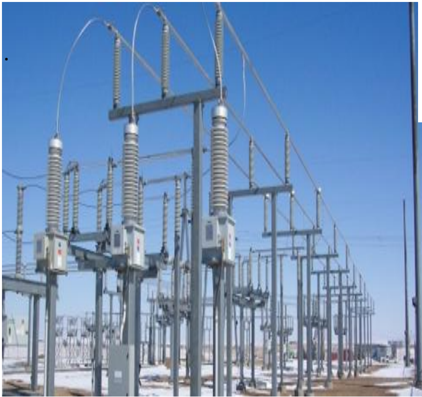
The electrical substation in the 1800 block of Allen Street is similar to this one.
