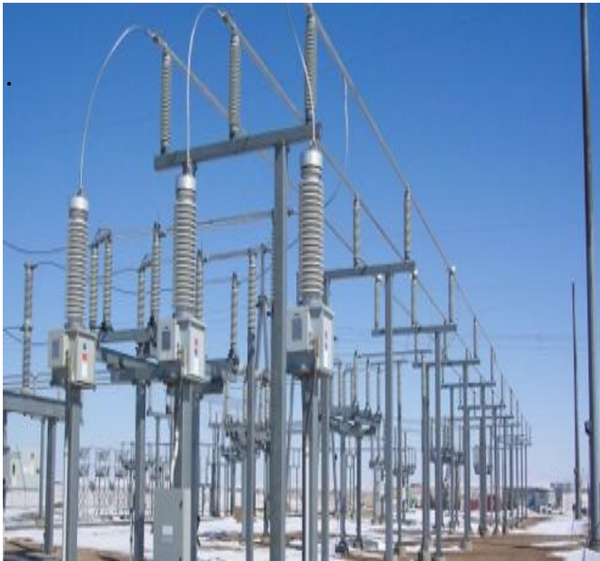
The electrical substation in the 1800 block of Allen Street is similar to this one.
