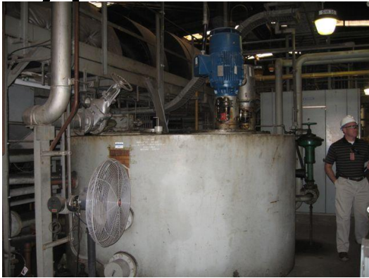
Lube Oil System
