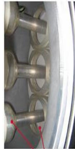
Earthing switch open
