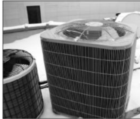
Air conditioning systems
